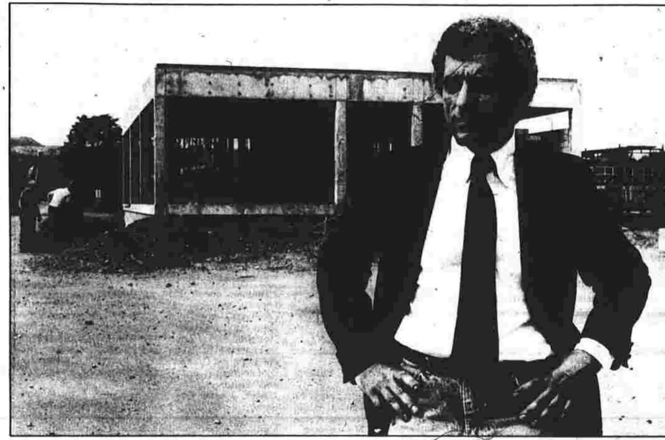
MR. MAYOR — Manchester Mayor Peter P. DiRosa Jr. today stands in front of crews working on the secondary part of the town's sewage treatment
